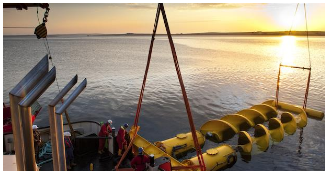
Fig. 5. Hydro-kinetic ASG installation (City University of Hong Kong, 2017).
