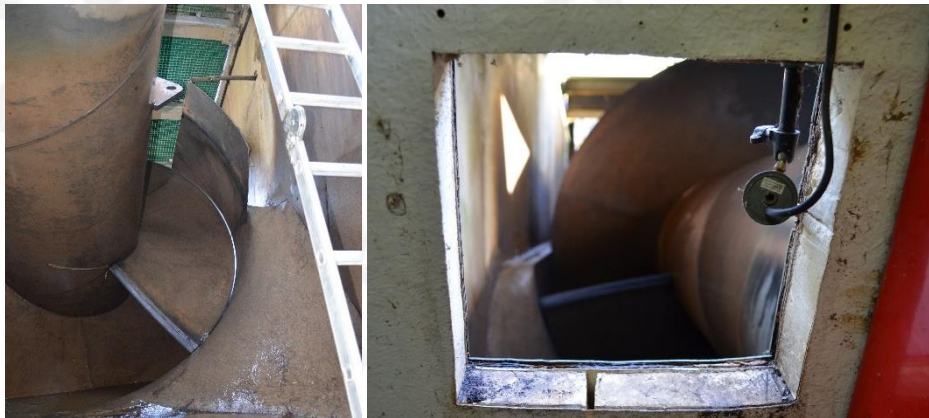
244 Figure 6: measurements were taken inside the screw's forebay for reference with upper water level measurements. Note in 245 the left image (a) that the baffle on the upper right side of the trough extends past the screw. The right image (b) 246 demonstrates monitor camera placement for tracking inlet water level and bucket filling.
