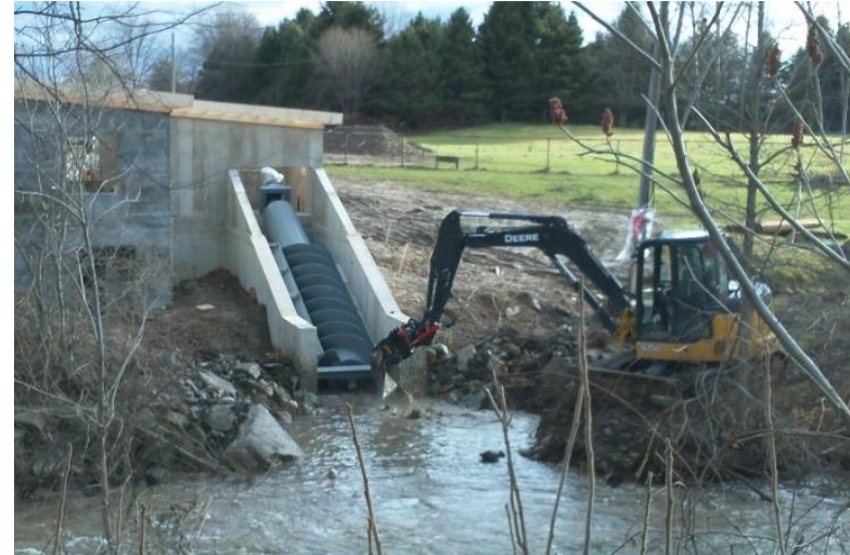
Fletcher's Horse World – ASG installation. (Greenbug Energy Inc., 2012)
